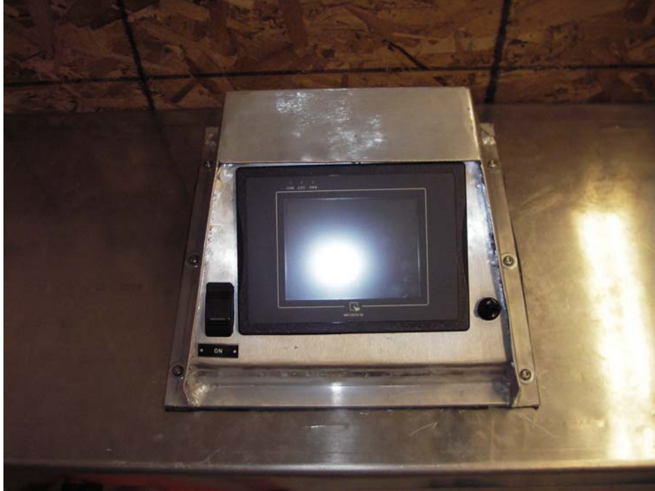
Figure 11 - Battery Management System LED Touch Screen
