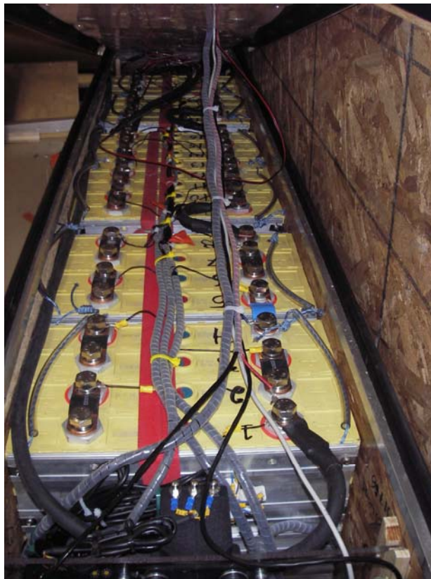
Figure 10 - Batteries and Controller Wired Inside Box
